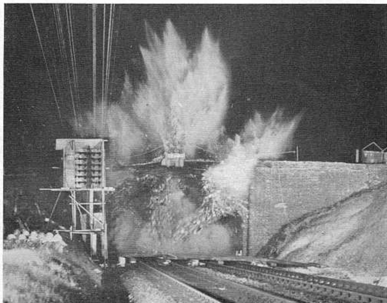
Bridge 179, carrying Quay Lane, being demolished by explosives on November 10. It will be replaced by a new bridge spanning three tracks
