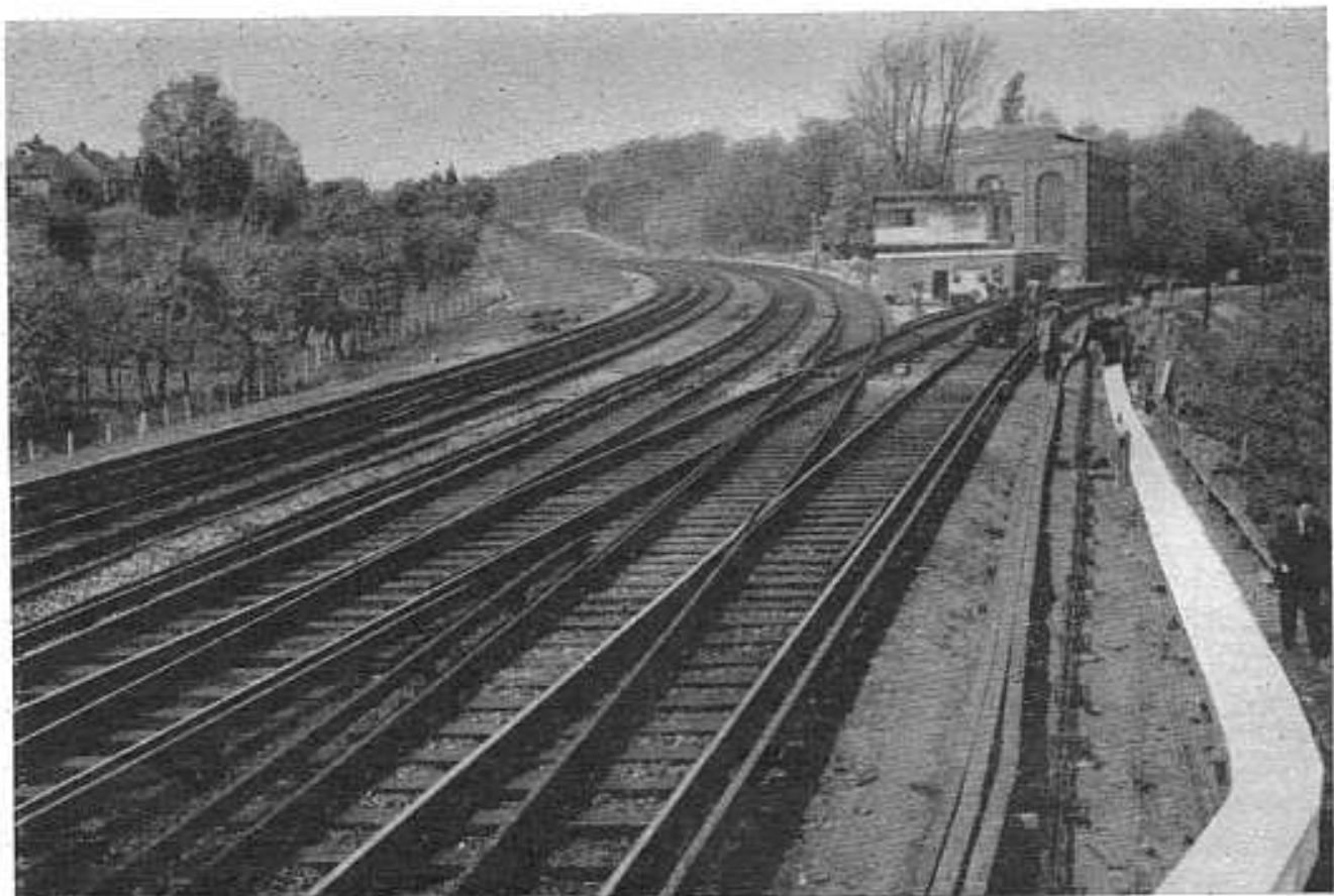
New junction at Shortlands, with the Catford Loop (on the right), laid on September 6-7, 1958
