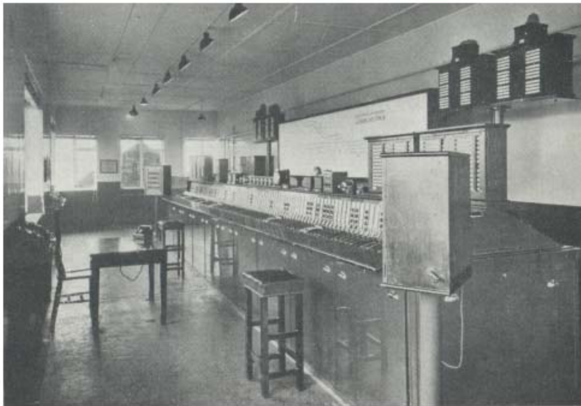
Interior of the new signalbox at Clapham Junction, showing the lever frame and the illuminated diagram
